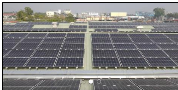
Figure 6. Building solar panels
